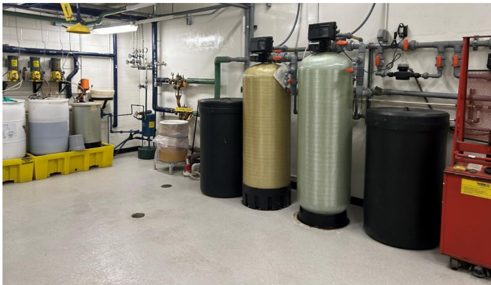
Fig 5. UW Stout Heating Plant water purifying room. Photo by Author on 29 November 2023.
