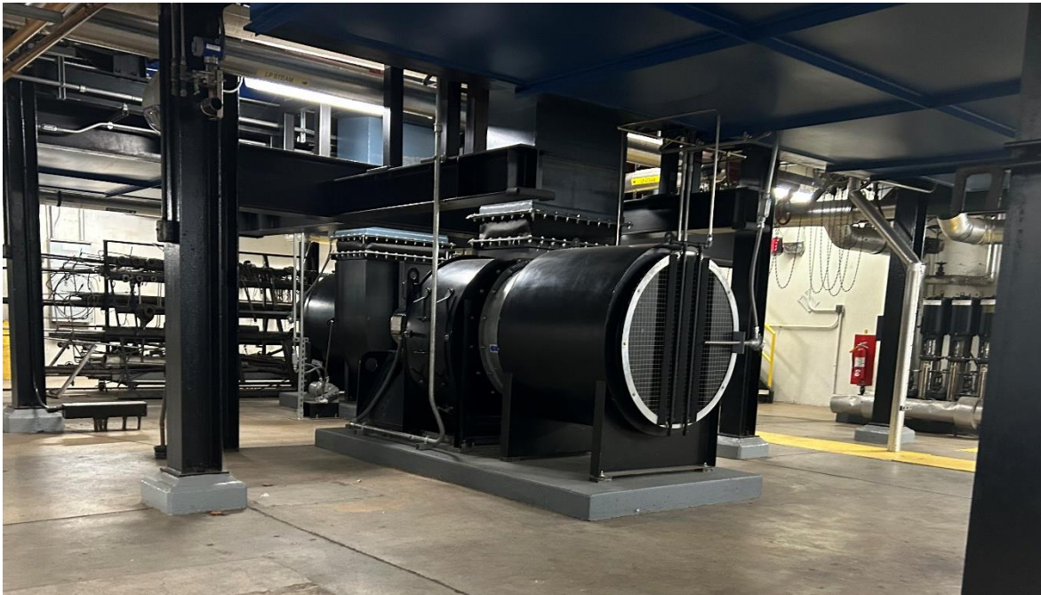
Fig 4. UW Stout Heating Plant basement room. Photo by Author on 29 November 2023.
