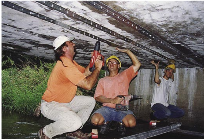
Workers installed SAFSTRIP® on this bridge in Edgerton, Wisconsin, using the MF-FRP system. The load rating for the bridge increased from HS-17 to HS-25 as a result.
