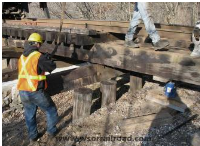
Figure 6: Rehabilitation of a timber bent for a bridge on the WSOR line in the Reedsburg subdivision. The deck was jacked up, and any deterioration in the piles was removed by sawing their tops off. A new pile cap is shown being placed over the piles. In the case of bridges which are double capped, a second pile cap would be stacked with the first (Wisconsin & Southern 2008).
