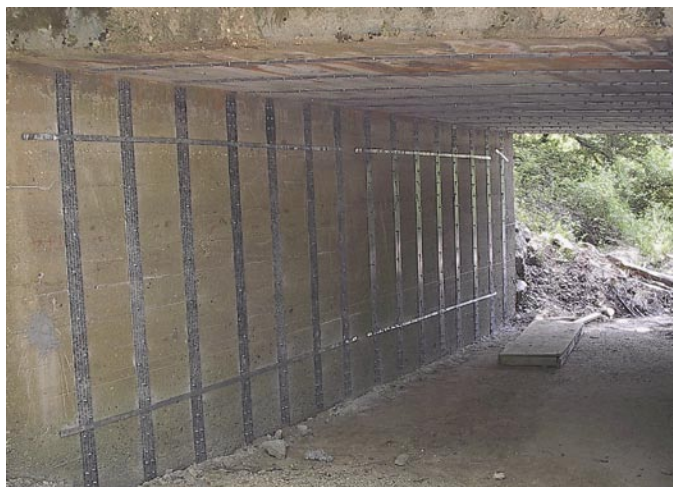
The abutment and deck of this bridge in Phelps County, Missouri, was strengthened using SAFSTRIP®.
