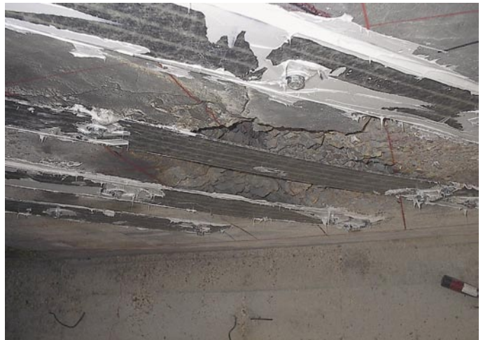
Severe deterioration prevented the application of a bonded strengthening system to this bridge in Pulaski County, Missouri, but MF-FRP applied SAFSTRIP® was able to repair the bridge.
