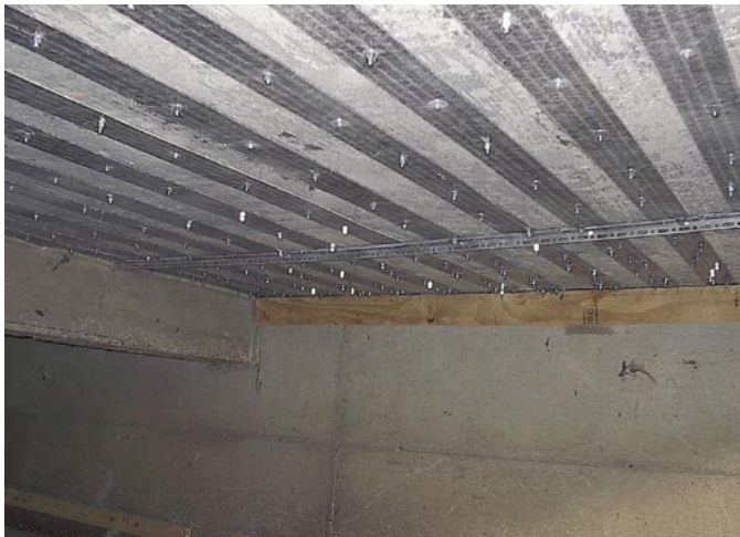
This bridge, located in St. James, Missouri, was load posted at the time of strengthening. After mechanically attaching SAFSTRIP® with concrete wedge bolts and anchors, the bridge load limit was raised to 20 tons.
