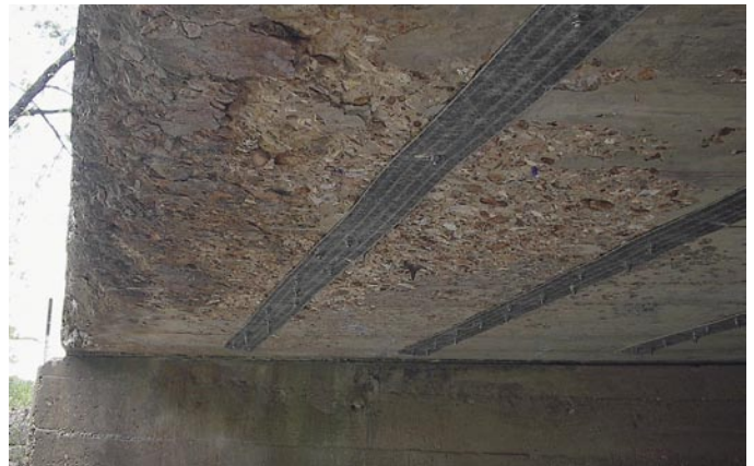
As a result of a SAFSTRIP® retrofit, the existing 12-ton load posting for this bridge in Phelps County, Missouri, was removed.
