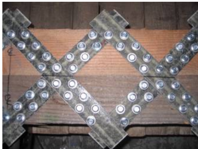
Figure 37: FRP strips attached before being trimmed. Each beam was 4" deep and the system was a total of 8" deep.
