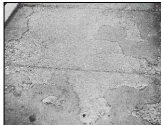
Figure 2-6 Scaling exposed on Concrete Surface. (Source: Photomac Construction industries, 2008)
