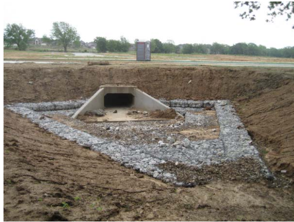
Figure 1-11 Riprap Basin to Protect Streambed and Stream Slope
