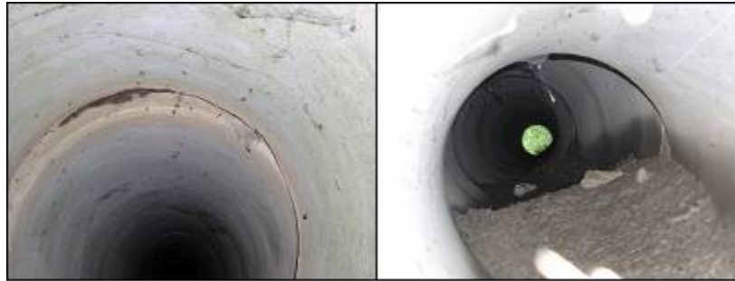
Figure 2-3 Culvert Pipe showing Cracks and Joint Separation
