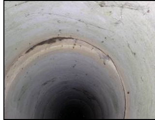
Figure 2-5 Transverse Cracks in a Culvert Pipe
