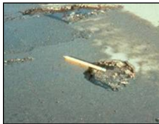
Figure 2-8 Spalling on a Concrete Surface. (Source: Caltrans, 2003)
