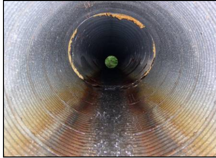
Figure 2-1 Corrosion in Culverts
