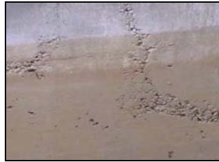
Figure 2-10 Honeycombing on a concrete surface. (Source: Department of Architectural Engineering, 2006)
