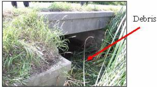
Figure 2-12 Debris at the Opening of the Culvert
