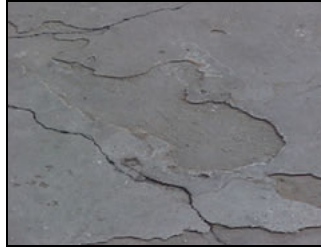
Figure 2-7 Delamination on a Concrete Surface. (Source: Concrete Restoration and Construction, 2007)
