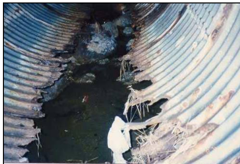
Figure 2-2 Deterioration due to Abrasion (Caltrans, 2003)
