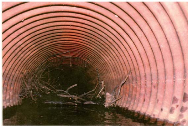
Figure 2-13 Beaver dam inside a culvert. (Patenaude, R., 2003).
