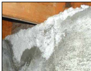
Figure 2-9 Formation of Efflorescence on a Concrete Surface.
