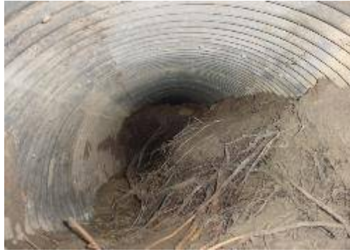
Figure 4-1 Example of Obstruction in Culvert (ASCE, 2008).
